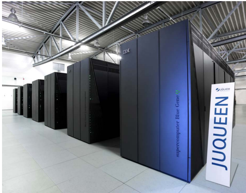
Figure 1: JUQUEEN at the Jülich Supercomputing Center.
